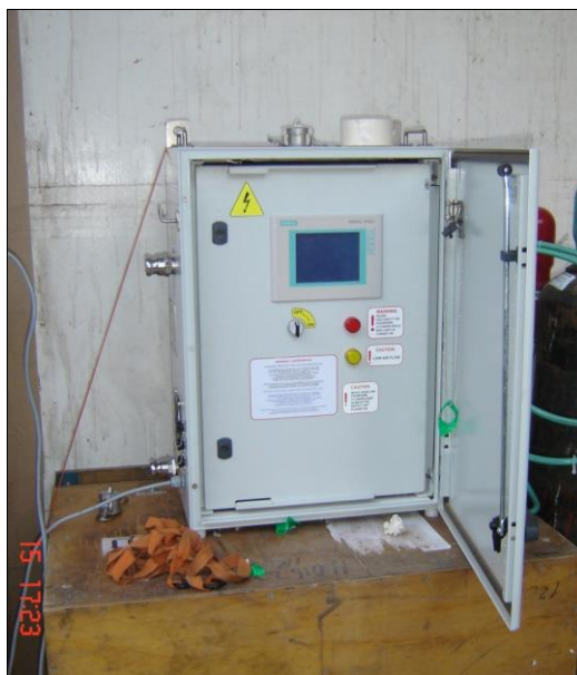
Picture 6. Horn Diluphos System, Model HDS 30 used for continuous phosphine injection.
